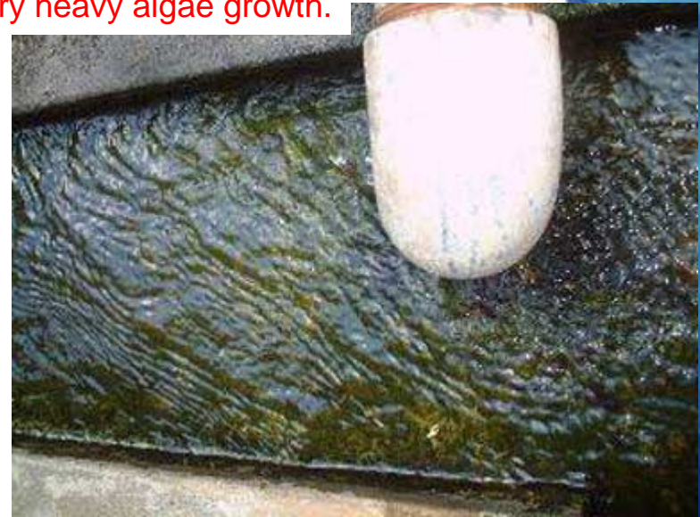
Drain stream of Cooling tower bleed
