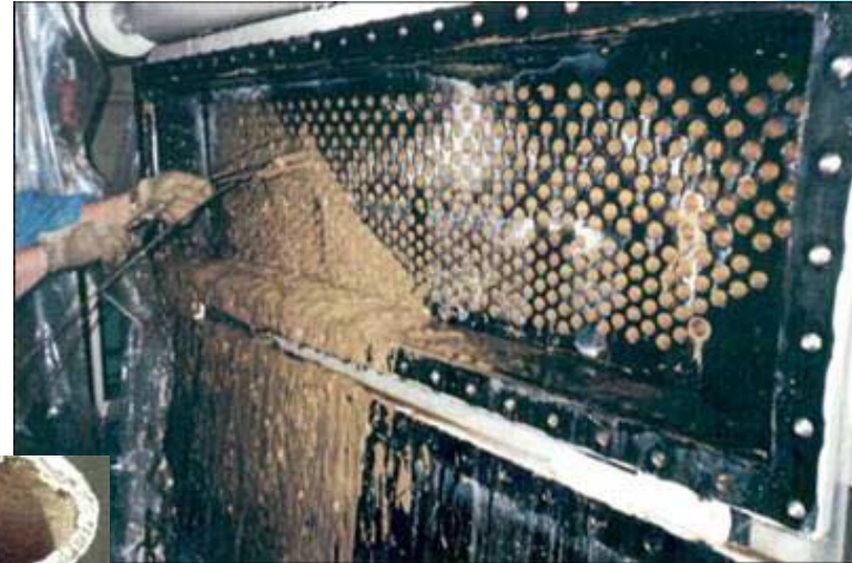
Heavily fouled Chiller condenser
