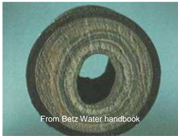
Heavily scaled pipe
