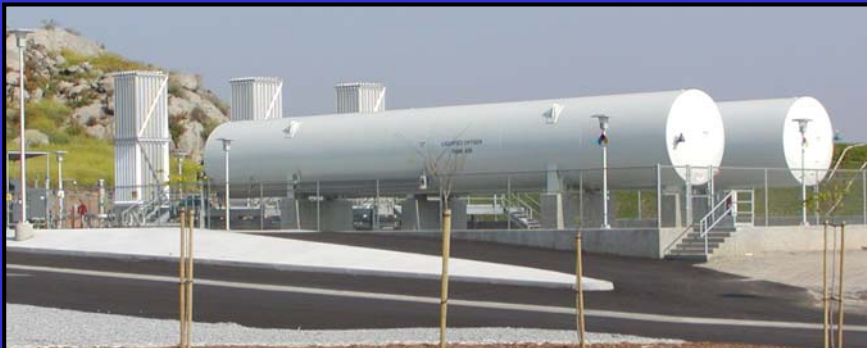
Liquid Oxygen Storage & Ambient Vaporizers
